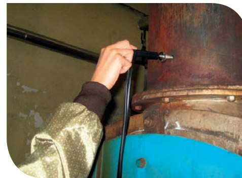
Picture 13: Measuring flue gases composition in the chimney.
