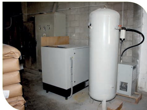
Picture 12: Compressed air system in a feedstuff factory.
