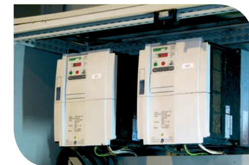
Picture 8: Variable speed drives installed.
