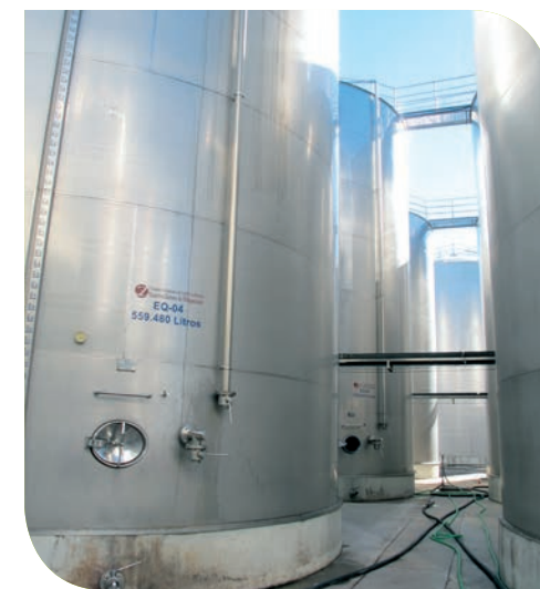
Picture 5: Refrigeration tanks in a winery.
