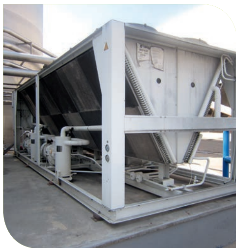
Picture 6: Cooling machines.
