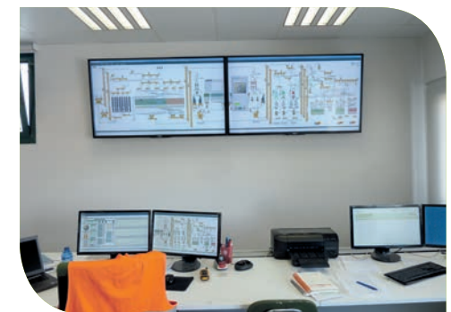
Picture 14: Control panel of the management systems.
