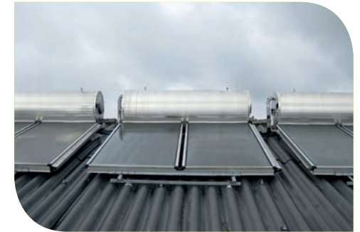
Picture 10: Solar panels for pre-heating water.
