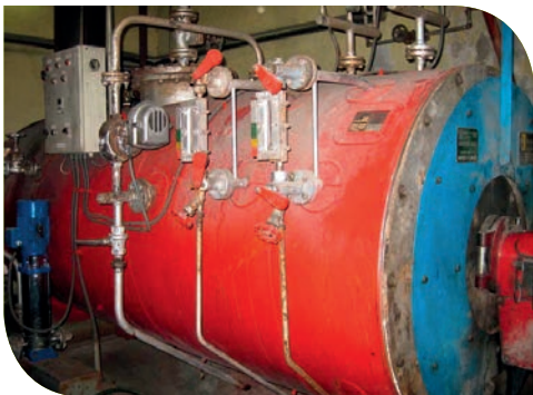
Picture 11: Diesel boiler.
