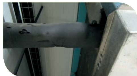
Picture 7: Damaged insulation in pipes.
